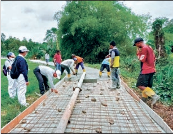
Tzu Chi Indonesia repaired a road for the village of Simpak in Parung Panjang, Bogor, Indonesia, to make it safer to use. The repairs took 20 days and were completed on November 15, 2021.
