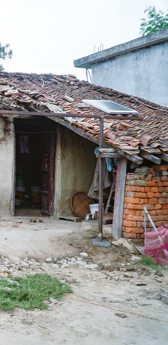
Srijana's home had a leaky roof. Volunteers stepped in to address this issue.
