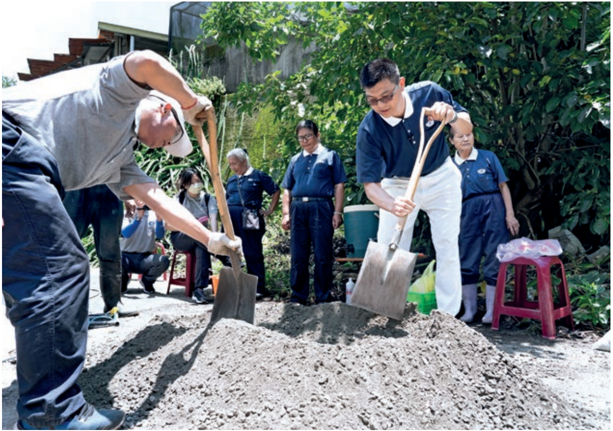
Cai (right) and other volunteers mix sand and cement to build some steps for a care recipient.
