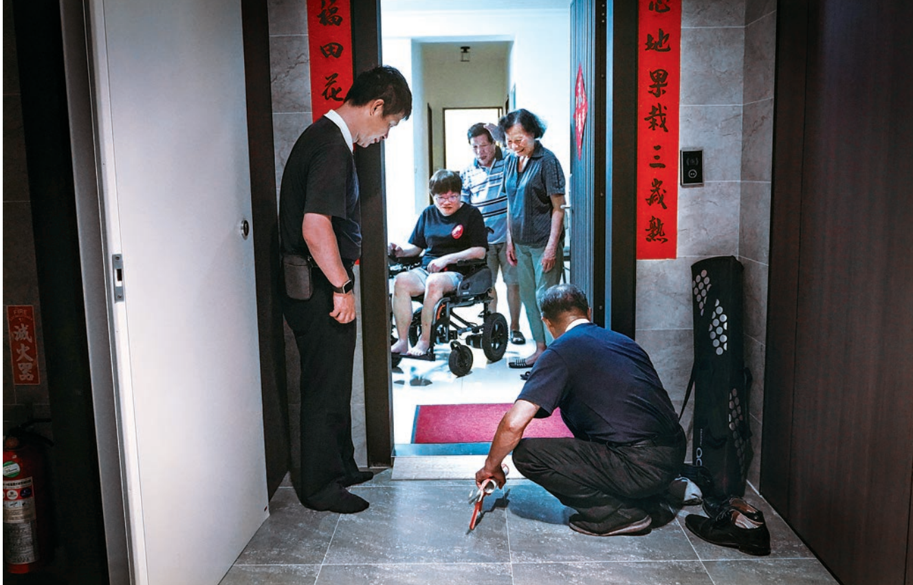
Yang Wen-zong (right) installs the completed threshold ramp at the entrance to Lin Jun-yi's home, making it safer for her wheelchair to navigate the height difference at the door.
